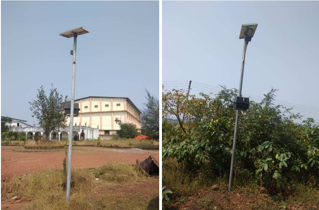
Solar Street Lights near Main Building and Ladies Hostel.
